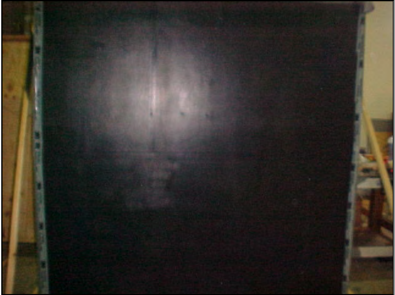
Photo No. 2 Control Wall All air seals on the exterior air barrier seal
