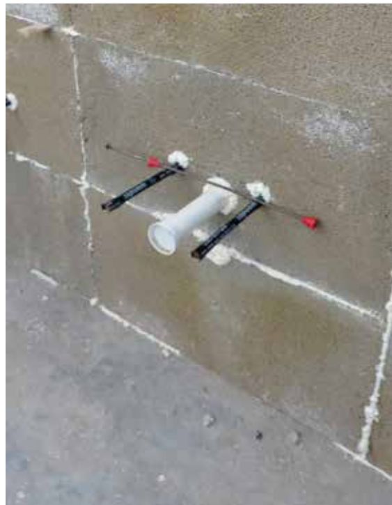
Figure 18: Mechanical items installed in Bautex Wall
