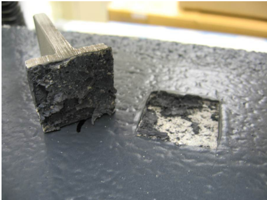
Photo No. 2 Pull-Off Strength - CMU Substrate Typical Condition After Testing
